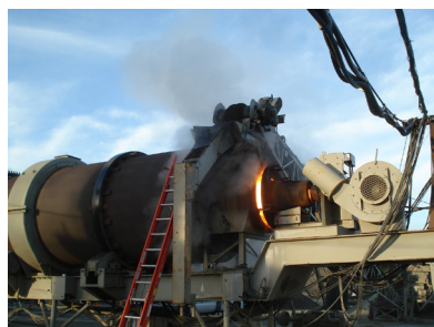
Of course you'd notice something this blatant during production. The problem is air system restrictions causing blow-back of combustion gases. Get out there and get it fixed. Photo courtesy of Cliff Mansfield.
